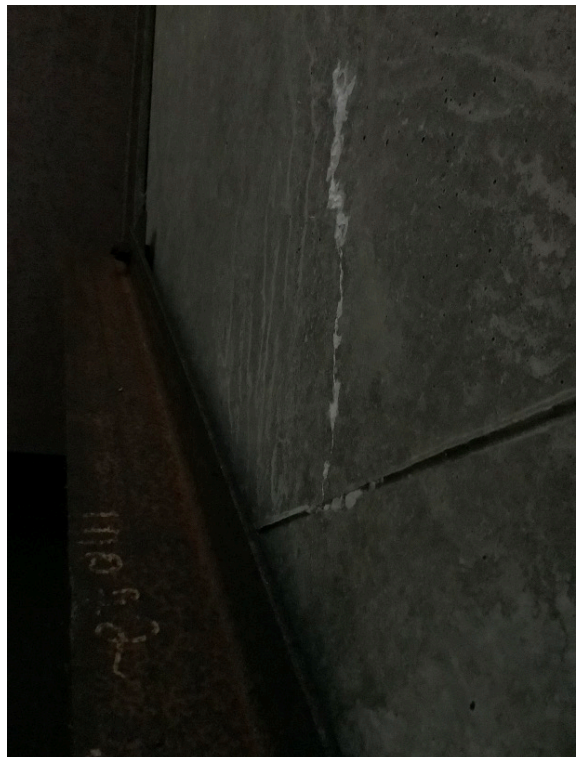
Efflorescence 2nd panel from right
